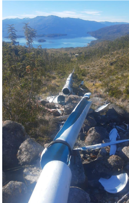
Figure 9 | Broken MCH pipe. Photographed by Gloria Baigorrotegui, February 2019.
