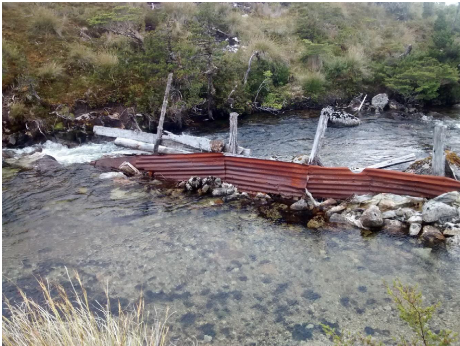
Figure 8 | Mini-hydro intake in Puerto Edén. Fondecyt MaReCe, November 2021.
