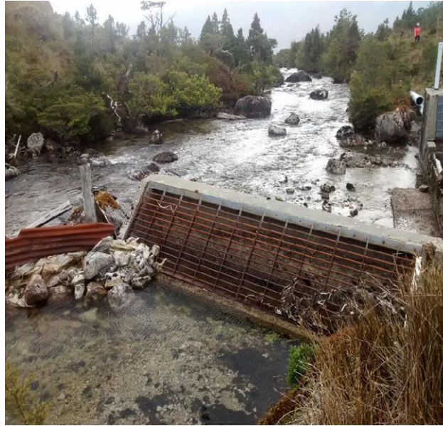
Figure 7 | Mini-hydro intake in Puerto Edén. Fondecyt MaReCe, November 2021.
