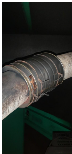
Figure 6 | Provisional patch that has become definitive for the wood-burning heater at the school. Fondecyt MaReCe, November 2021.
