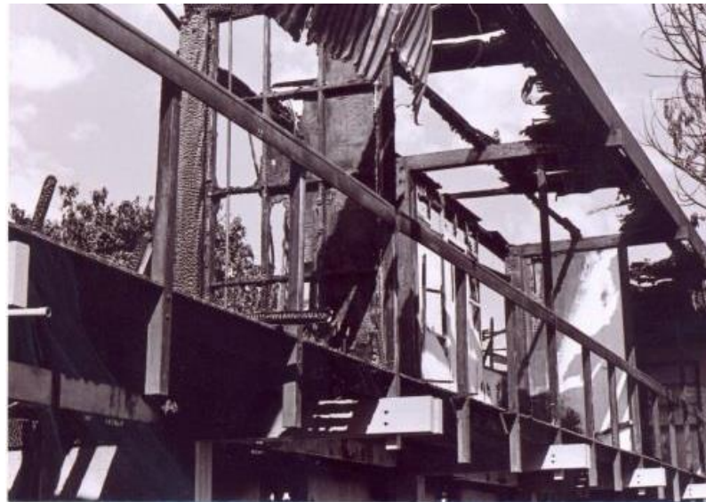
Figure 12: OCA I after the fire.
