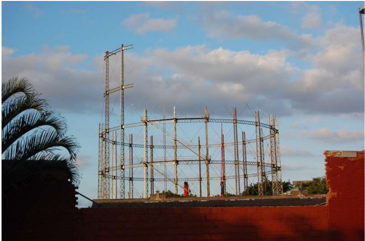
Figure 3: May 2017, the process of dismantling the gas tank in Rio's São Cristóvão neighbourhood.
